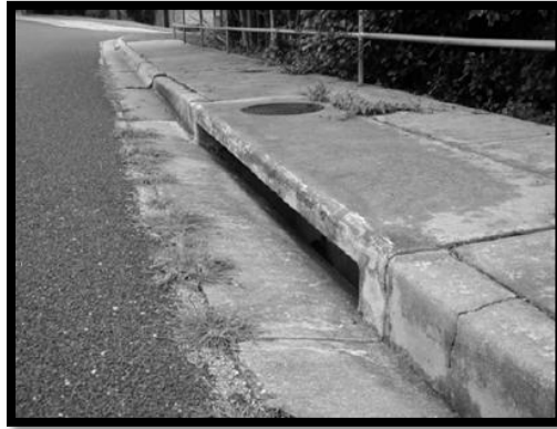
Figure 4. Curb inlet for stormwater system directly connects street to creek
